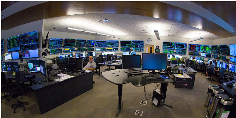
Figure VII.3: Control room of SLAC as an example for the HBS central control room [Dir23].
