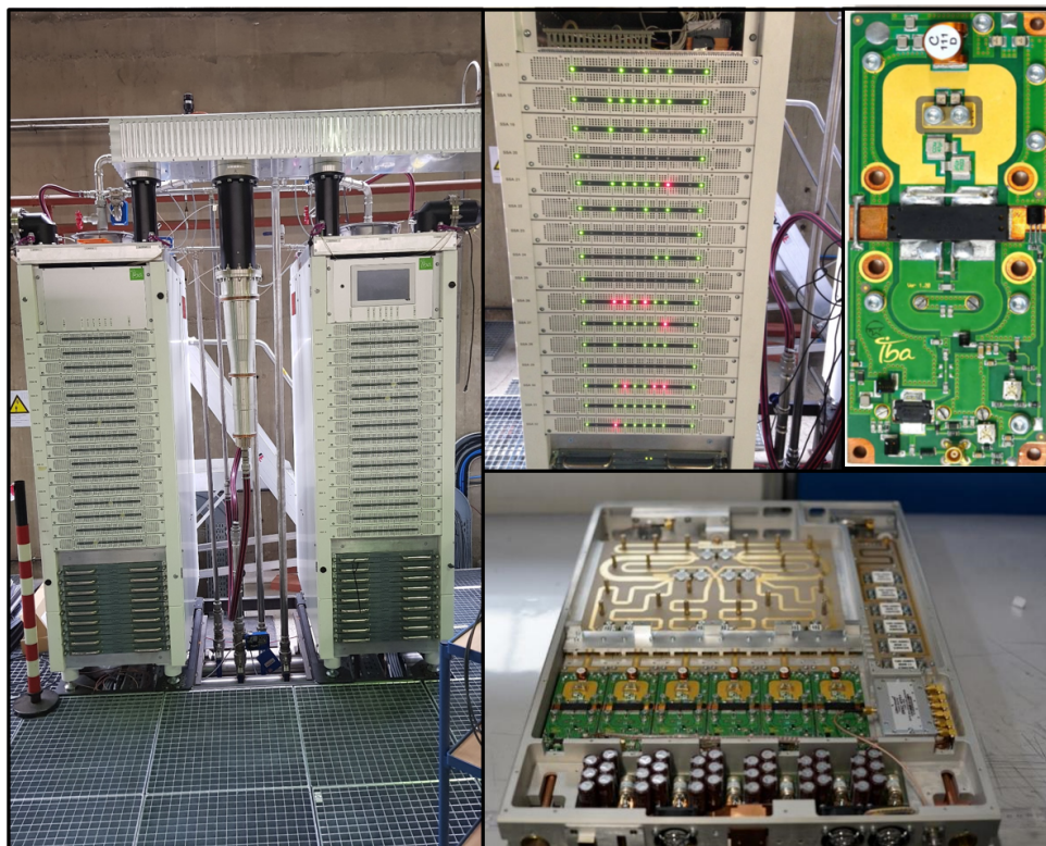
Figure IV.1: 192 kW, 176.1 MHz Solid State Amplifier (SSA) developed for the MYRRHA project.
