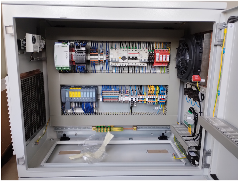
Figure II.65: One of the decentral control racks for the target handling tool.
