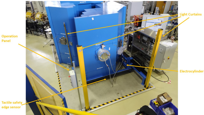
Figure II.64: Safety sensors at the shielding gate.
